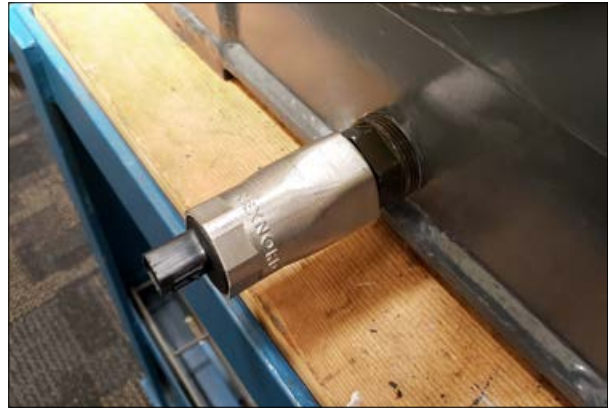
Figure 12 – Completed installation of oil quality sensor
