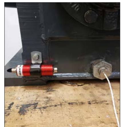
Figure 8 – Converter Installed on A+Plus Drive on end of drive
