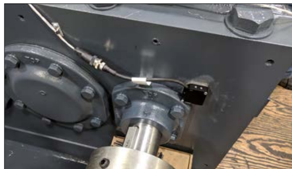
Figure 4 – Installed vibration sensor
