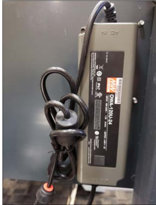
Figure 16 – Power supply for Edge Device installed on back on mounting plate
