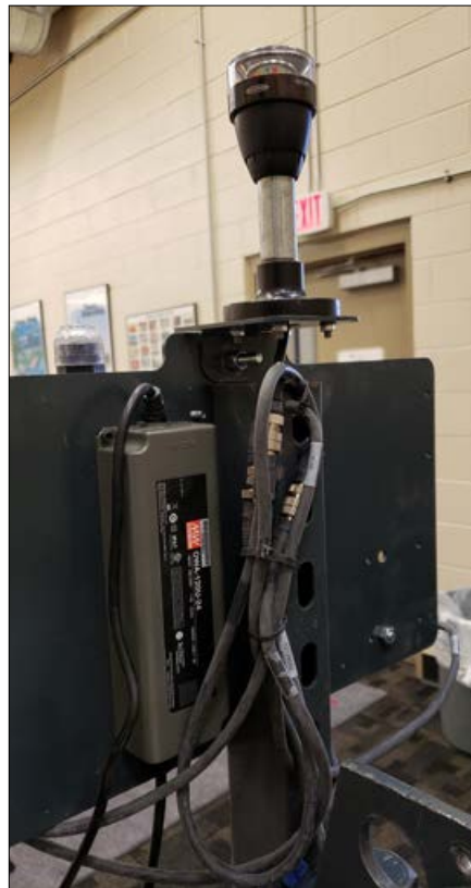
Figure 25 – Excess cable coiled and secured to the back of the Edge Device mounting plate
